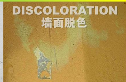
细纹裂缝 HAIRLINE CRACK
